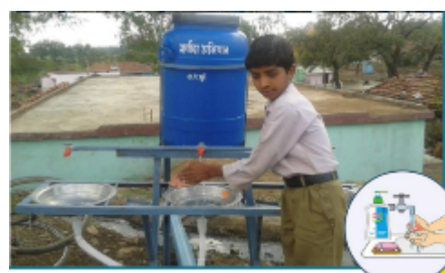
Figure 34: COVID-19 sensitive handwashing unit installed in a school
