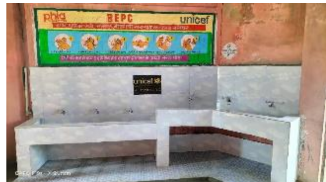
Figure 11: Group handwashing facility with COVID sensitive elbow tab installed, in a school from Patna district, Bihar
