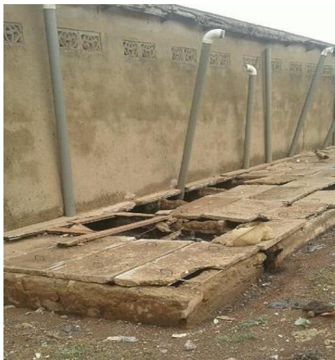
Figure 44: Damaged KVIP/VIP public toilet
