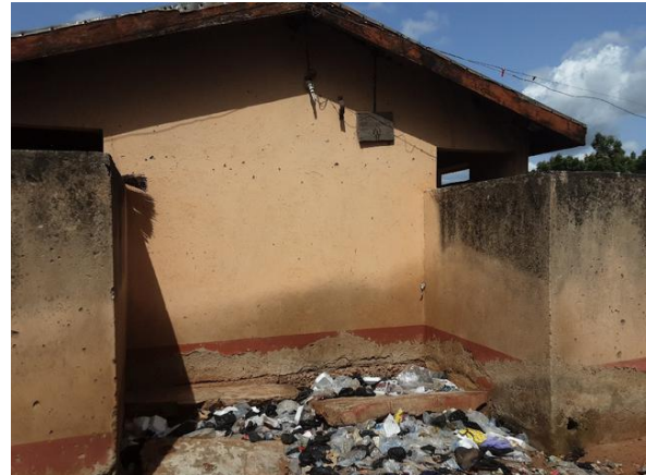
Figure 43: Public toilet containment filled with solid waste
