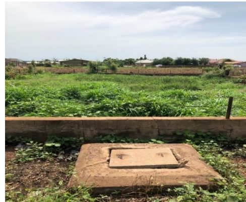
Figure 7: Constructed wetland connected to the SSNIT septic tanks
