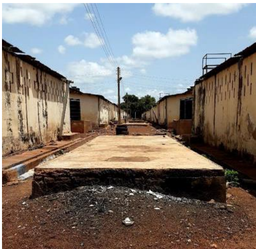
Figure 12: Image of multiple centralised septic tanks at Police barracks (CRS, 2021c)
