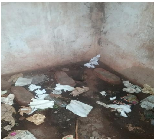
Figure 40: Filthy slab at a public toilet
