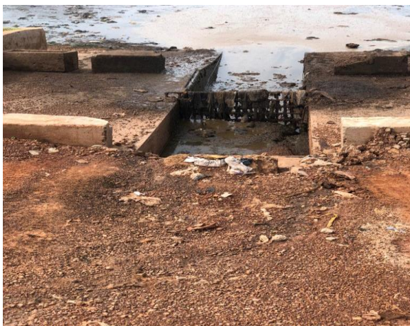
Figure 18: Installed grit chamber for truck discharge
