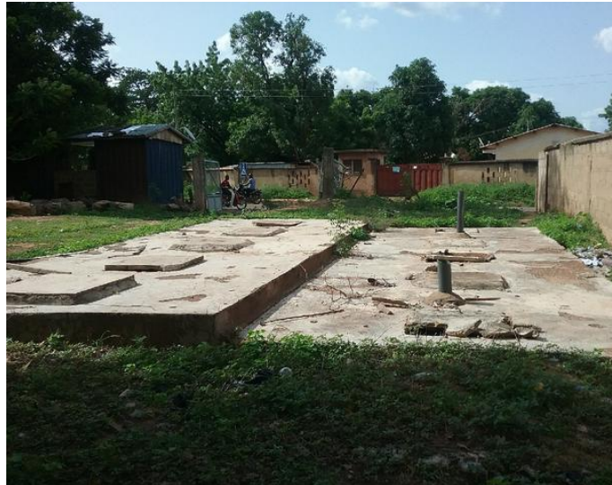
Figure 47: Centralised septic tank at the SDA hospital
