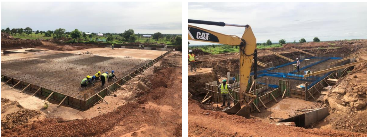
Figure 20: Ongoing works for new 1000 cum capacity FS treatment plant at the Gbalahi landfill site
