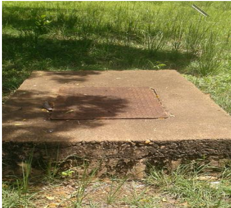
Figure 11: Image of a septic tank at Kamina barracks (CRS, 2021c)
