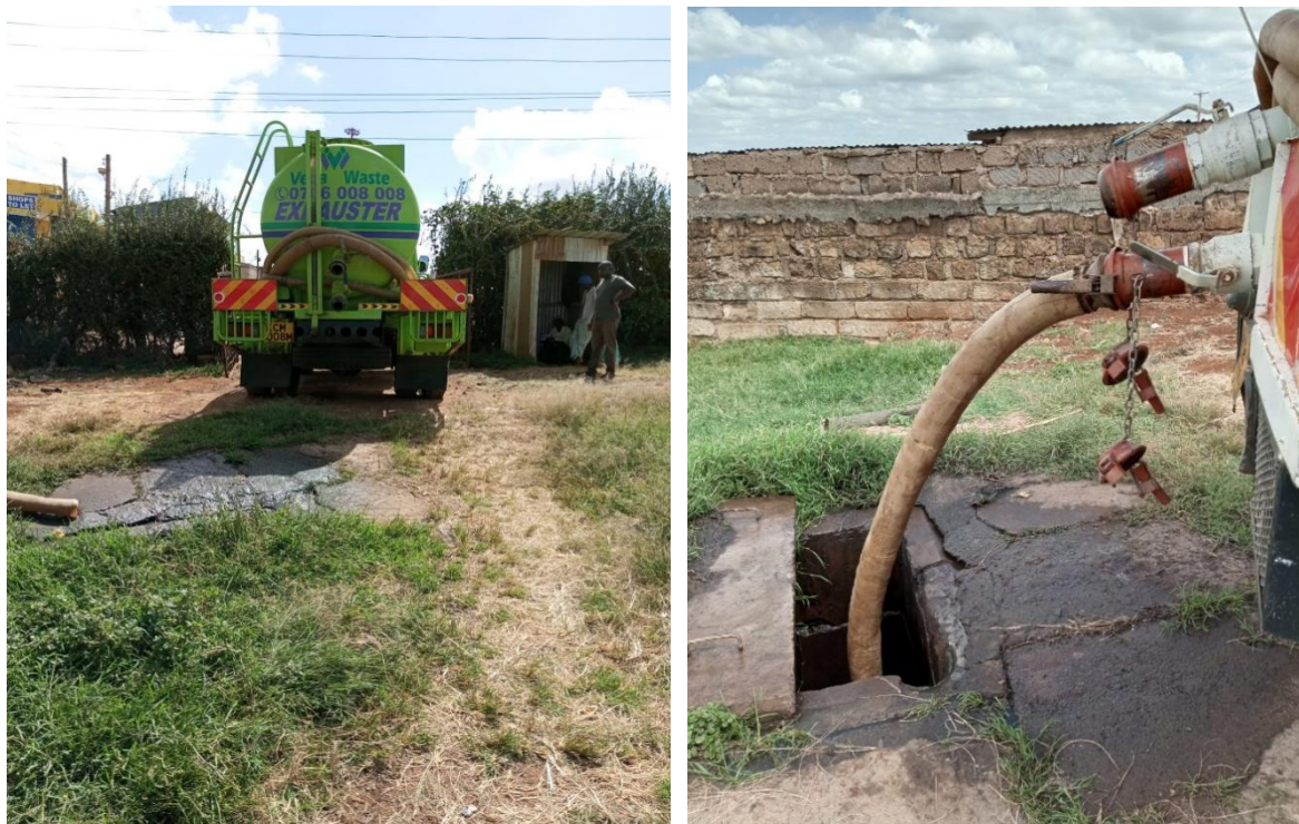
Figure 3: Vacuum trucks emptying faecal sludge to sewer plant at Gakoromone (June 2022).
