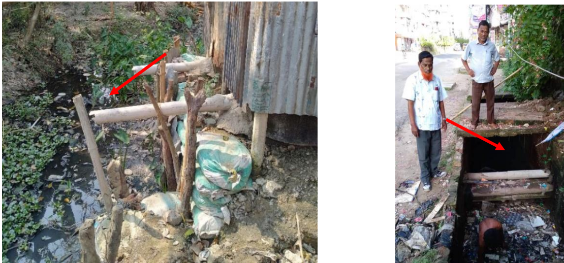
Figure 6: Containment technologies and their connections in Feni. Left: Toilet Pit open to a nearby water body, Right: Toilet pipe connected to open environment (Source: Feasibility study 2020-21/DPHE).
