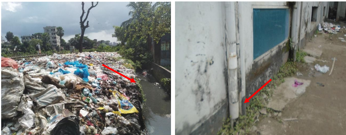
Figure 6: Containment technologies and their connections in Gazipur. Left: Toilet Pit open to a nearby water body, Right: Toilet pipe connected to open environment. (Source: Feasibility study 2020-21/DPHE).
