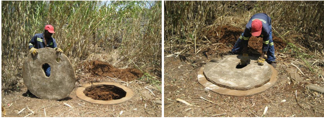
The ring beam is made in concrete and the pit dug down inside to a depth of between 1m and 2m. The firmer the soil the deeper one can dig
