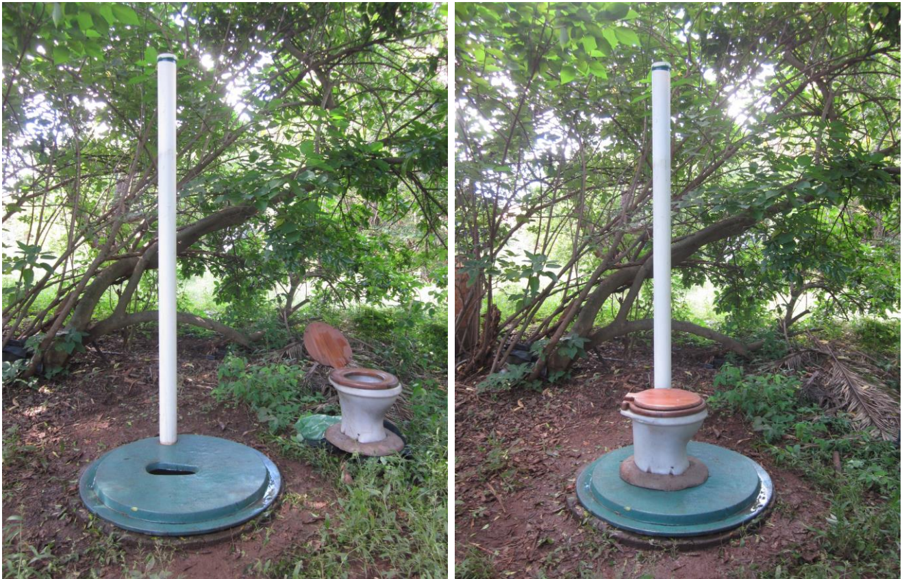
The arrangement of a fibreglass slab and pedestal and 110mm pipe fitted made by Prodorite. These are fitted over a ring beam and shallow pit.
