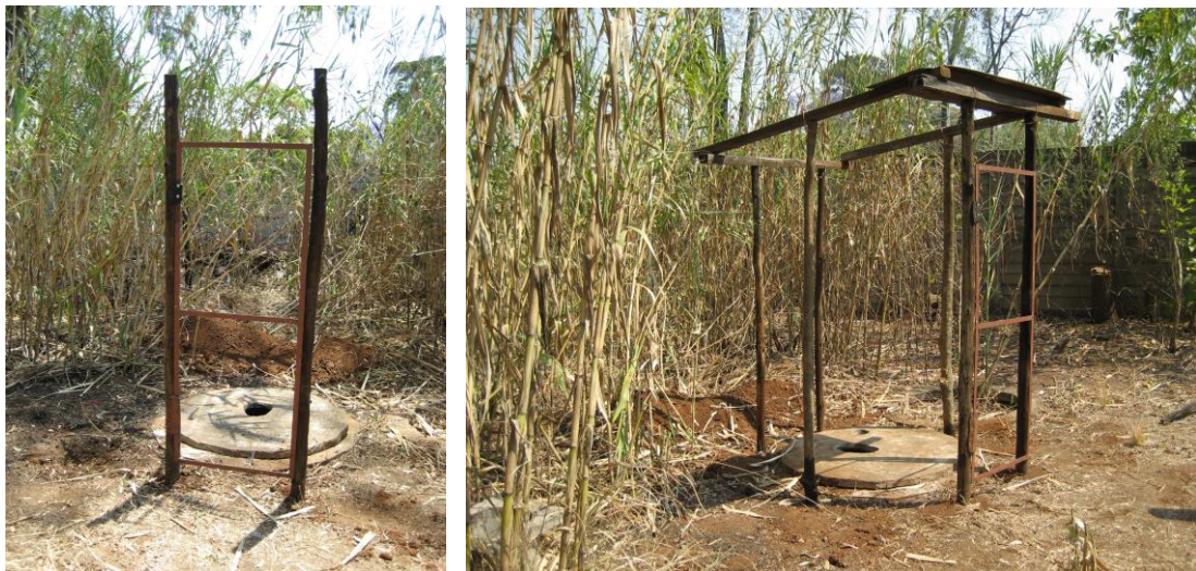
Poles are used as uprights and should be treated against termite attack. A steel door frame can be made and suspended on car tyre rubber hinges or strong metal hinges.
