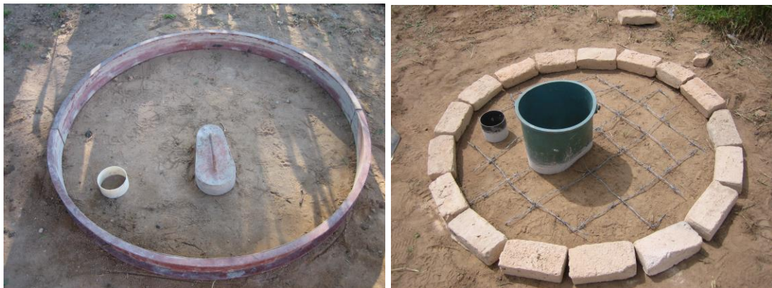
However such moulds may not be available so the standard method uses bricks
