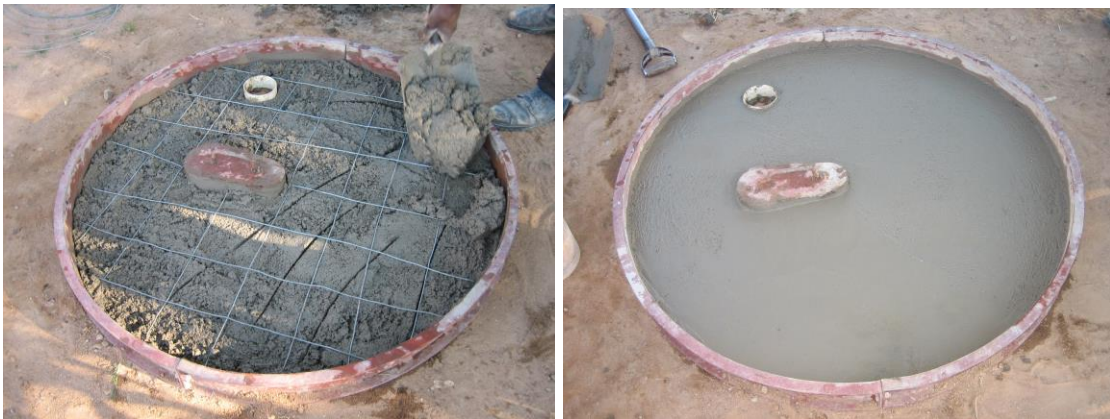
Steel moulds were used in this case to cast the slab and make the squat hole
