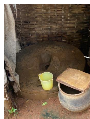
Figure 8: Pit latrine connected to unlined pit (Source: Dimple Behal/CSE).
