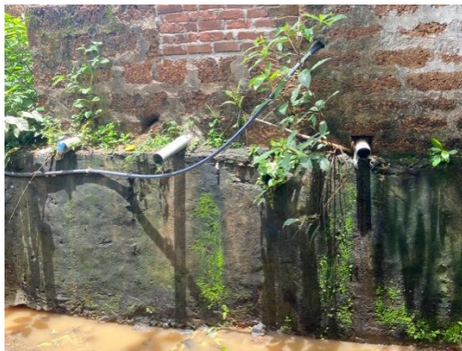
Figure 9: Containment Outlet in Open Drain (Source: Dimple Behal/CSE).
