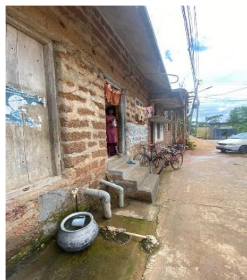
Figure 7: Septic tank connected to open drain, Ward 3 (Source: Dimple Behal/CSE).
