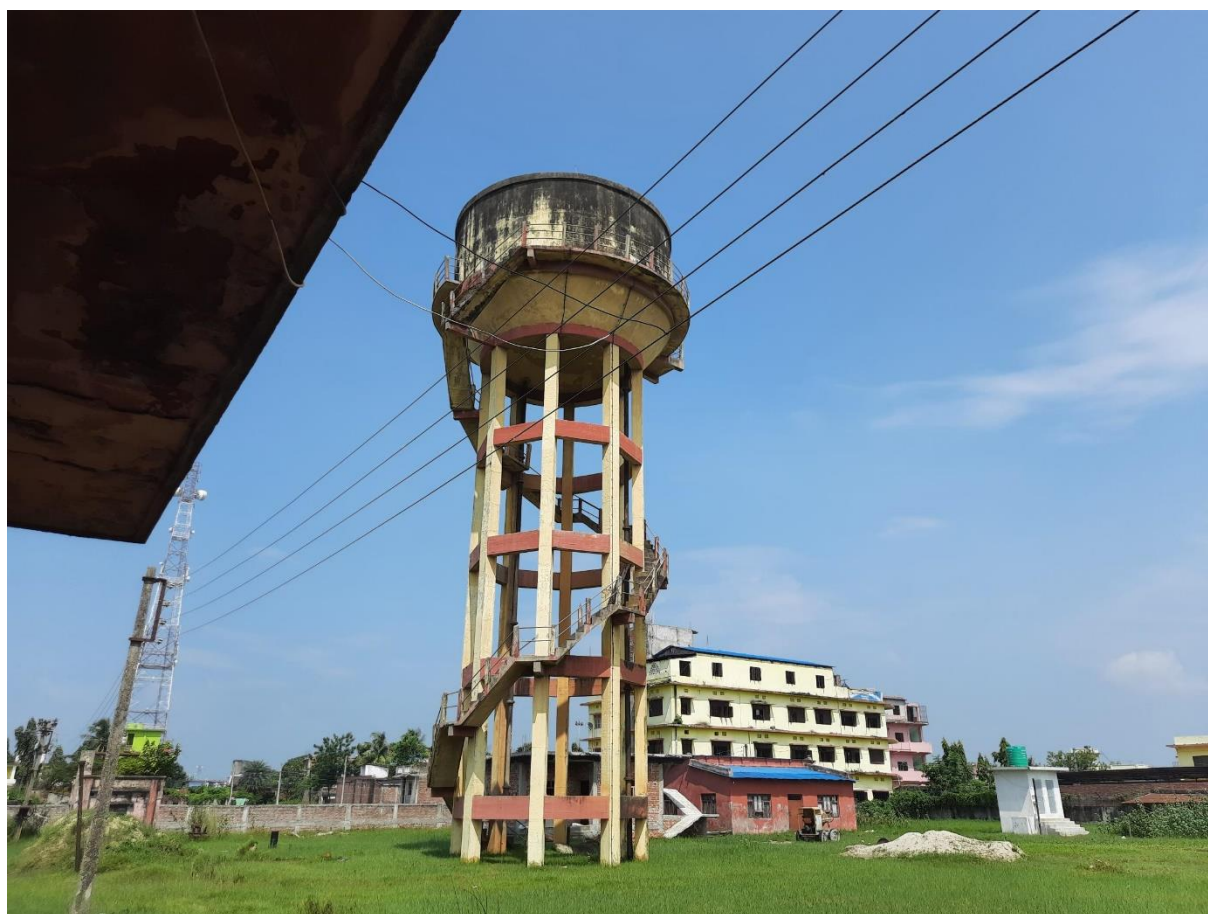
Figure 15: Overhead Tank for Piped Drinking Water Supply System in Siraha Municipality.
