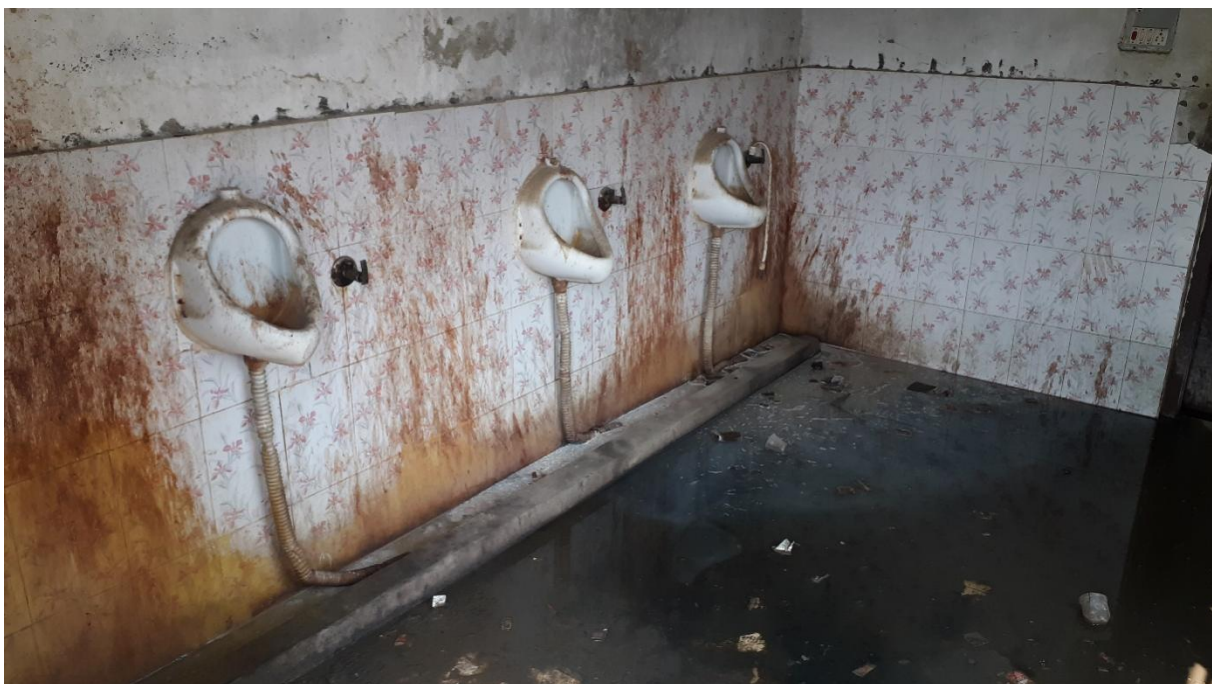
Figure 9: Overflowed urinal of the public toilet.
