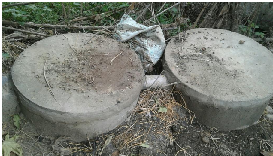
Figure 4: Inappropriate design of the twin pits.
