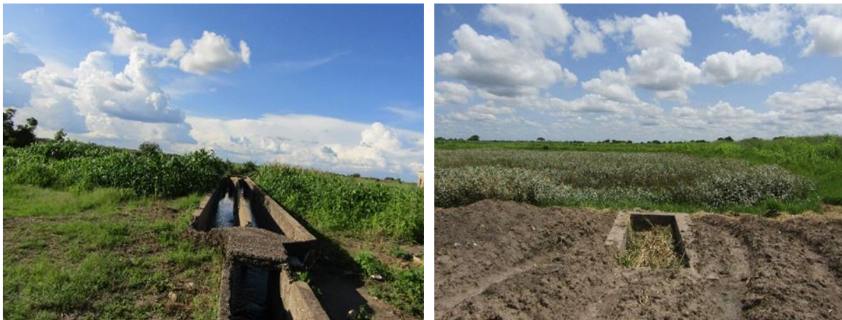
Figure 5: Evidence of blockages and leakages in the systems. LHS: Clear sewage devoid of suspended solids reaching the Natuseko Ponds; RHS: The Old Ngungu Ponds with completely no flows. (Source: Author).
