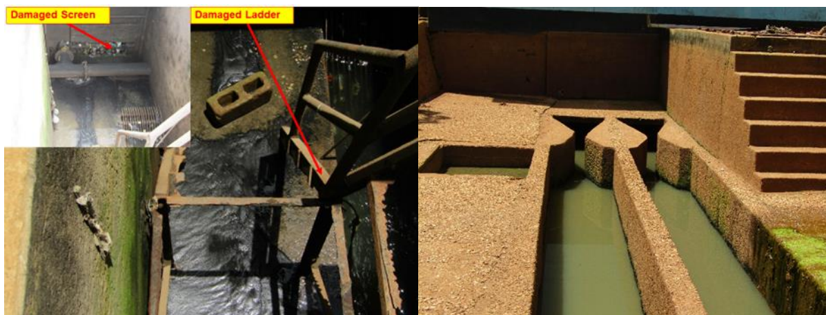
Figure 4: State of selected sewage pump station in Kabwe. LHS: PS1 Sewage Pump Station showing a damaged access ladder to the inlet chamber and an insert of a damaged screen; RHS: PS2 Sewage Pump Station with flooding inlet channel during a period of ZESCO power outage (no standby power supply (Source: Author).
