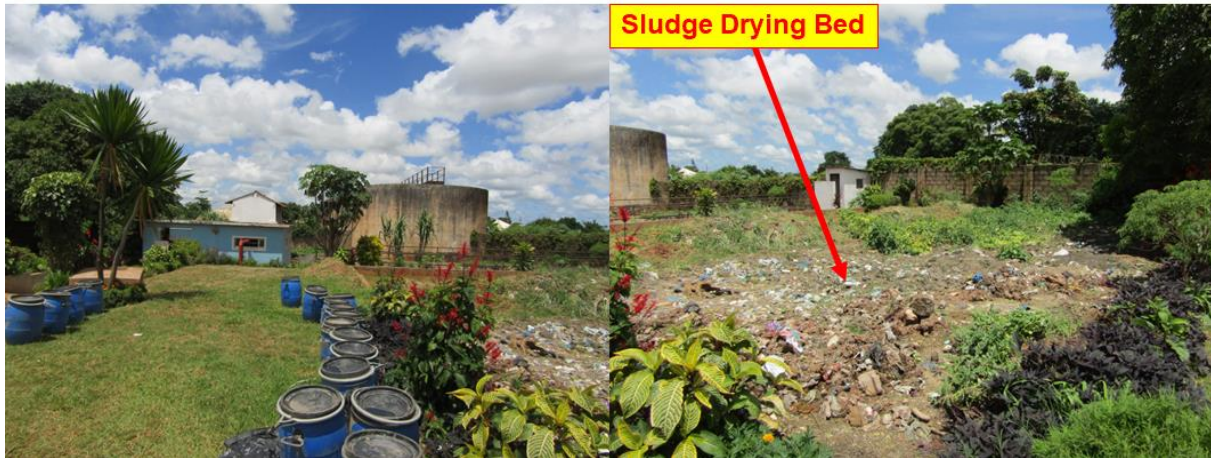
Figure 9: Faecal sludge emptying and treatment in Kabwe. LHS: Barrels used to transport emptied faecal sludge; RHS: The faecal sludge drying bed at PS2. (Source: Author).
