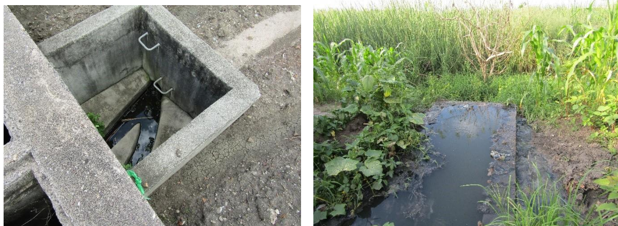
Figure 8: General state of sewage ponds in Kabwe. LHS: Blocked Old Ngungu inlet Channel; RHS: Natuseko Ponds overgrown with weeds and with a blocked the inlet. (Source: Author).
