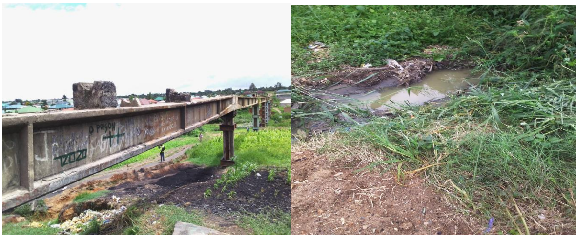
Figure 3: Collapsed sewer trunk main and wastewater ending up in the environment (Source: Author, 2022).
