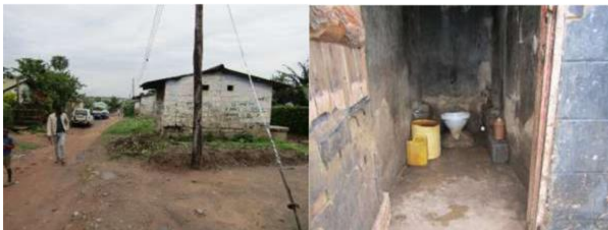
Figure 7: Communal Toilets in Mindolo Section D (LHS: Row of Communal Facilities; RHS: Inside one of the Toilets).
