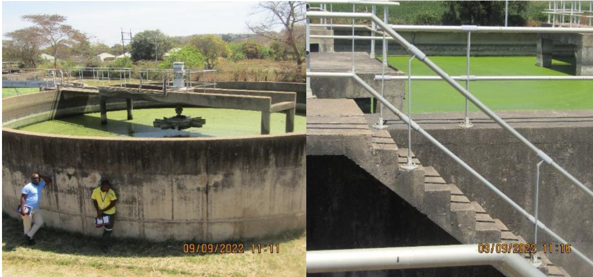
Figure 10: The state of the Primary and Secondary aeration tanks at the time of the site visit.
