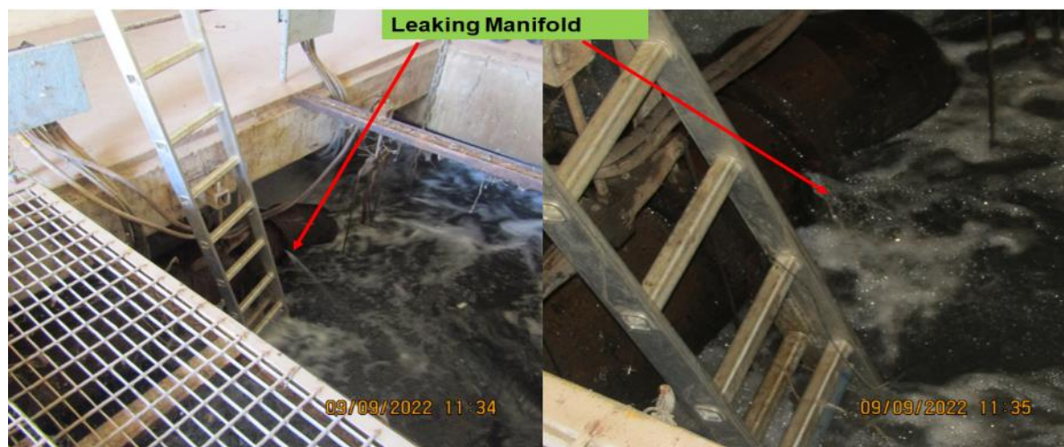
Figure 9: The damaged manifold in the receiving well at Chawama Activated Sludge WWTP.
