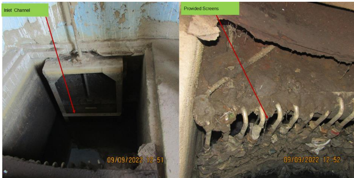
Figure 5: The Inlet Channel to PS 03 showing the coarse screens that have been provided.
