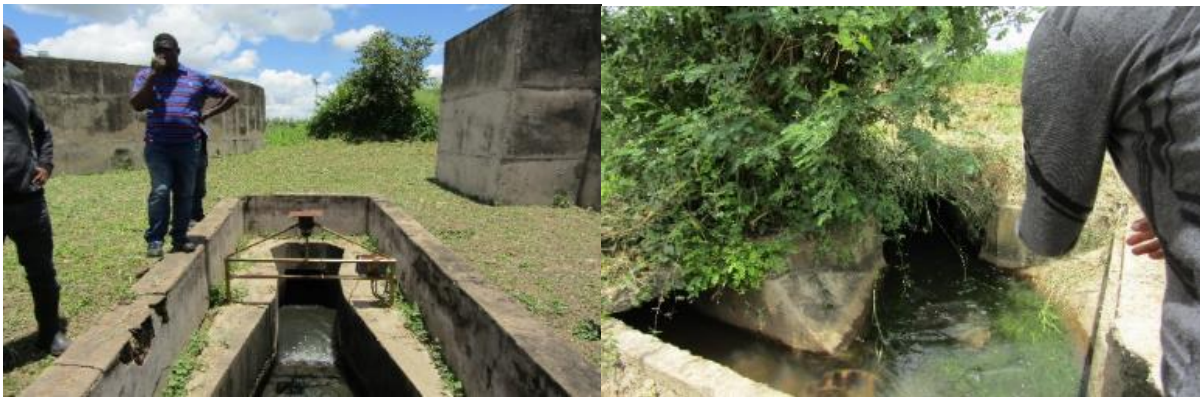
Figure 14: Evidence on lack of flow measuring devices at the WWTP (LHS: A dysfunction Partial Flume meant to measure the effluent from the activated plant; RHS: The outlet from the Maturation ponds with no flow measuring device).
