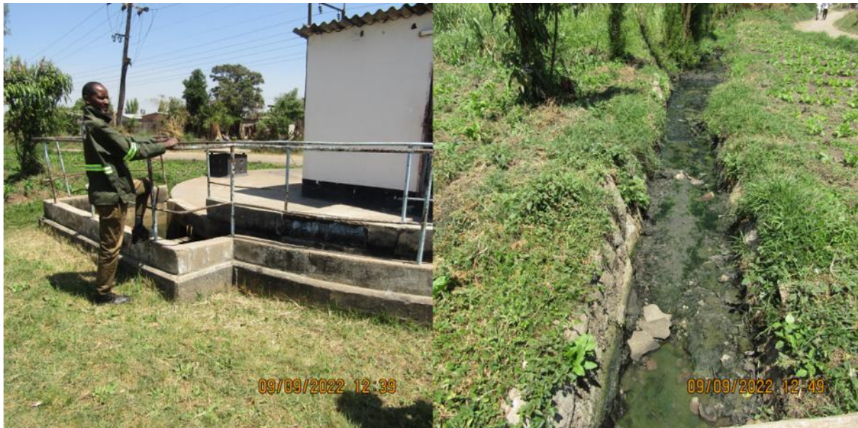
Figure 6: Pump Station No. 02 (Note bypass channel on the RHS with evidence of wastewater flow in it).
