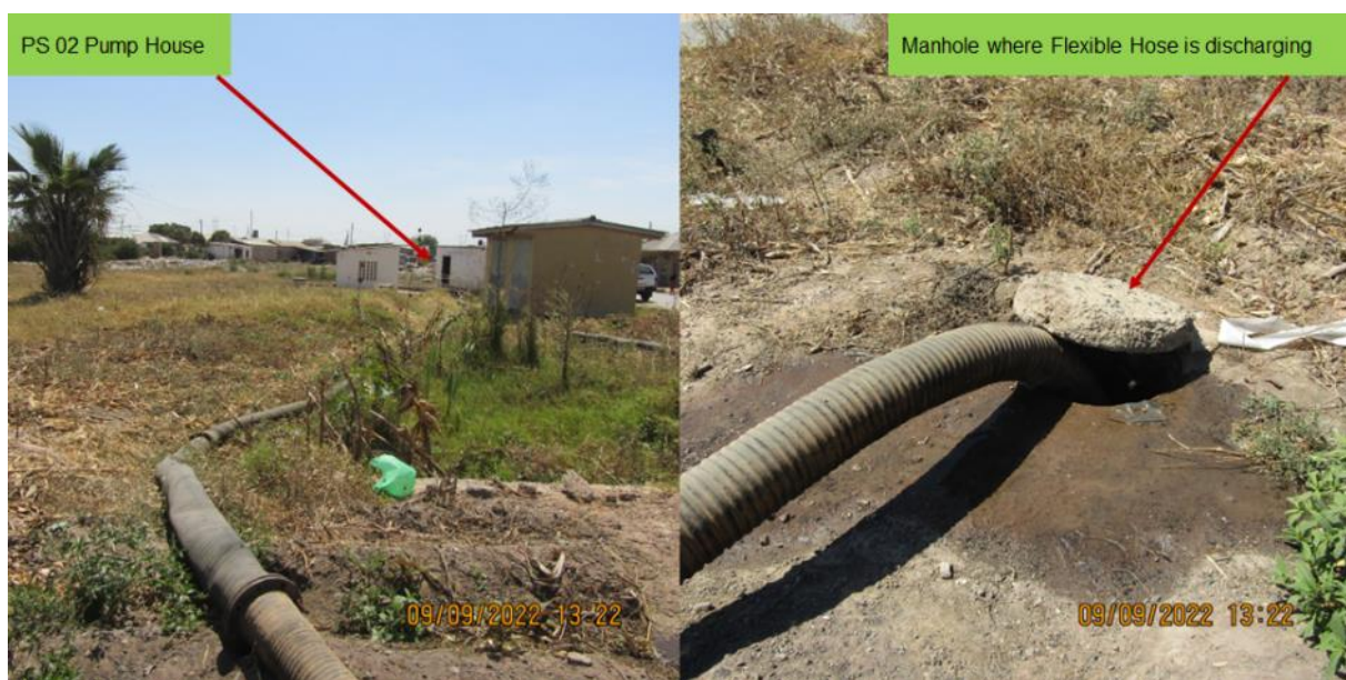
Figure 4: Pump Station No. 02 with the improvised flexible hose terminating at a manhole.
