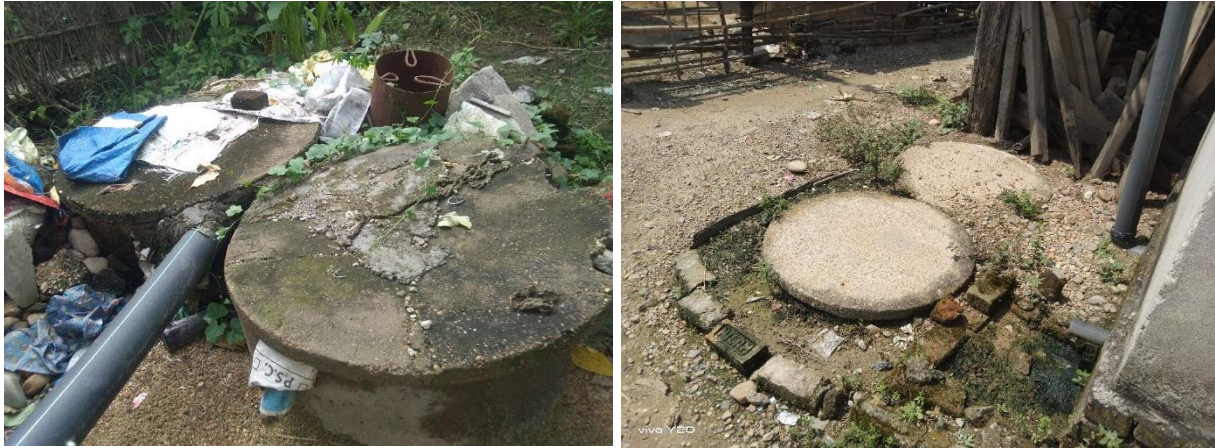
Figure 4: Inappropriate design of the twin pits.
