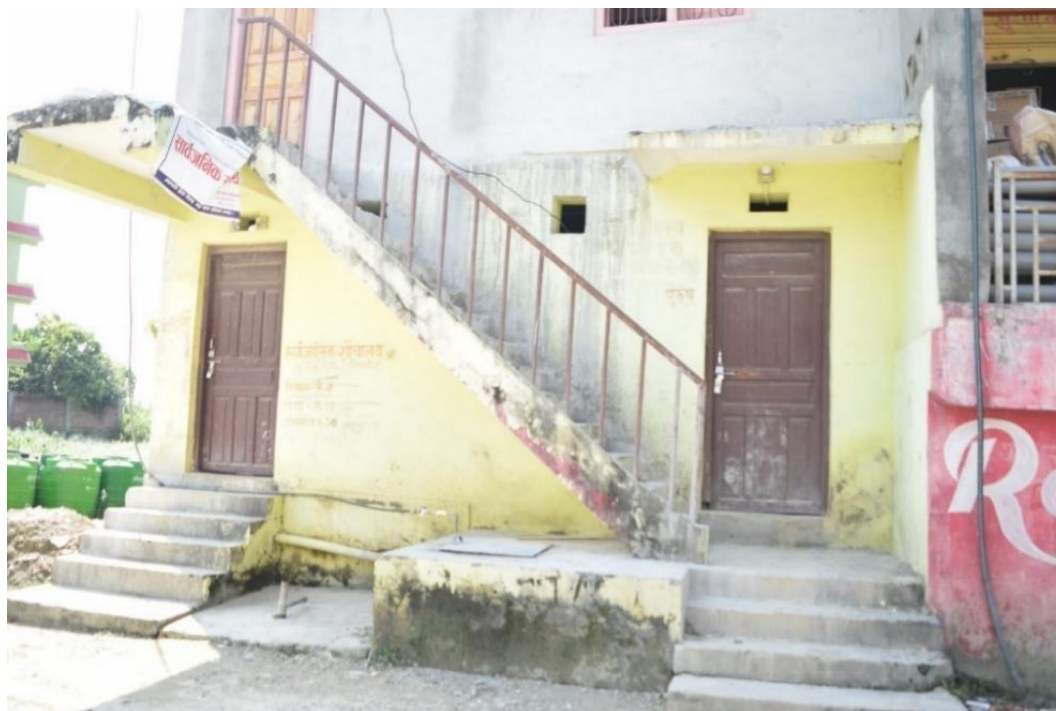
Figure 12: Non-functional public toilet at Katari chowk.
