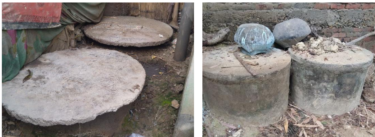
Figure 2: Inappropriate design of the twin pits.
