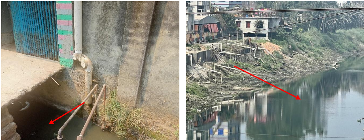
Figure 6: Containment technologies and their connections in Kaliakair Municipality. Left: Toilet outlet connected to open drain, Right: Toilet outlets direct connected to waterbodies. (Source: Field Survey 2023/ O.CREEDS_ WaterAid Bangladesh).
