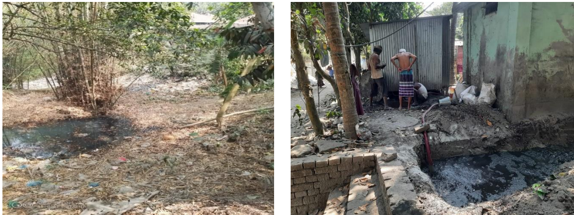
Figure 6: Containment technologies and their connections in Singair Municipality (Source: Field Survey 2023/ O.CREEDS_ WaterAid Bangladesh).
