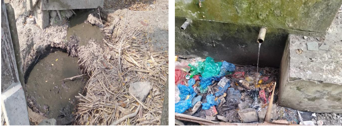
Figure 6: Containment technologies and their connections in Kalihati Municipality. (Toilet outlet connected to open drains) (Source: Field Survey 2023/ O.CREEDS_ WaterAid Bangladesh).
