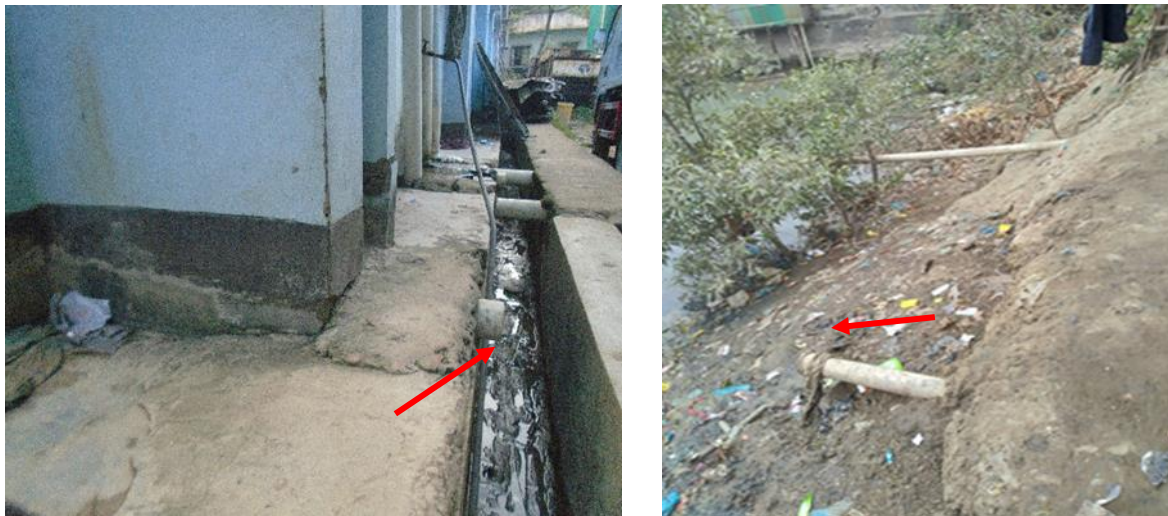
Figure 6: Containment technologies and their connections in Cox's Bazar. Left: Toilet Pit open to a nearby open drain. Right: Toilet pipe connected to open environment (Source: Feasibility study 2020-21/DPHE).
