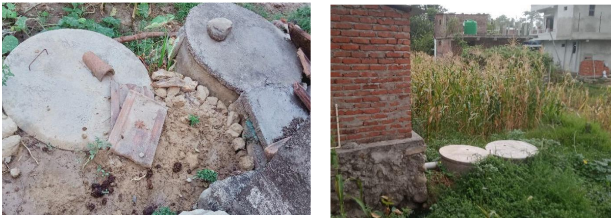
Figure 8: Inappropriate design of twin pits, where the distance between the two pits is less than 1.2m.
