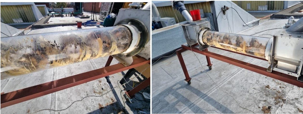
Figure 4.26. Synthetic sludge sticking to blades and side walls
