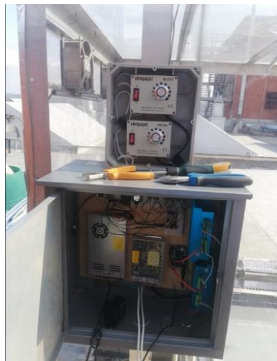
Figure 3.7. Electrical control boxes
