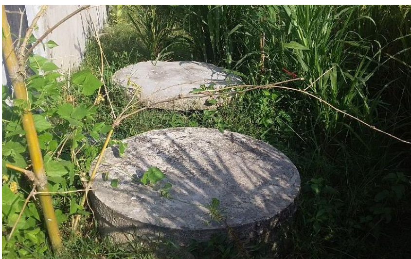
Figure 5 : Inappropriate design of the twin pits, where the distance between two pits is less than 1 m.
