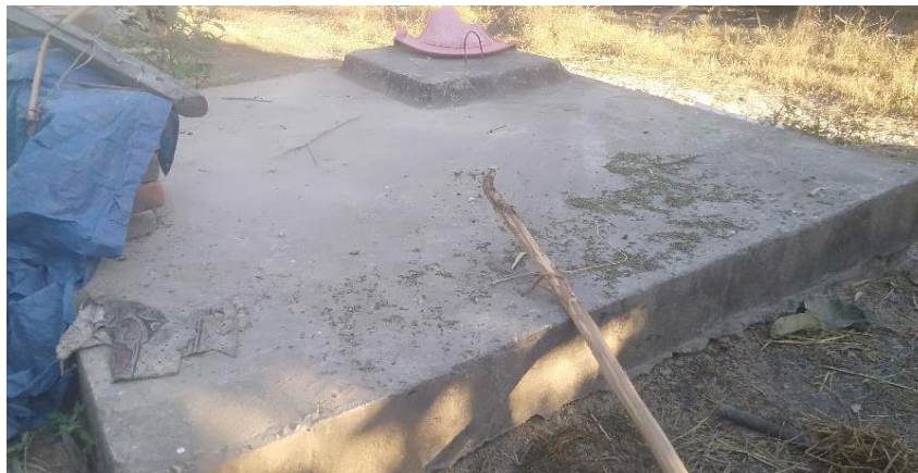
Figure 3: Fully Lined Tank.
