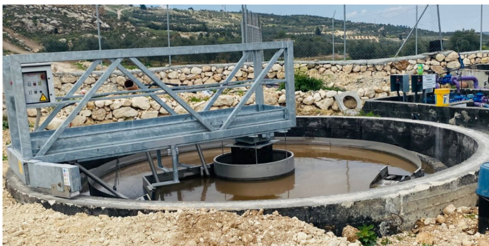
Figure 10: Picture of the WWTP of Kharas town (Clarifier).
