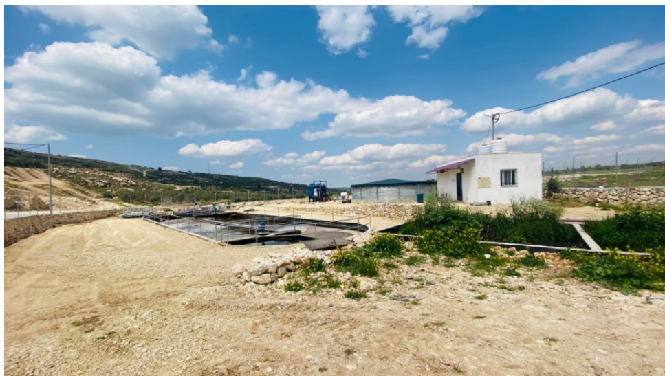
Figure 9: Picture of the WWTP of Kharas town (general view).
