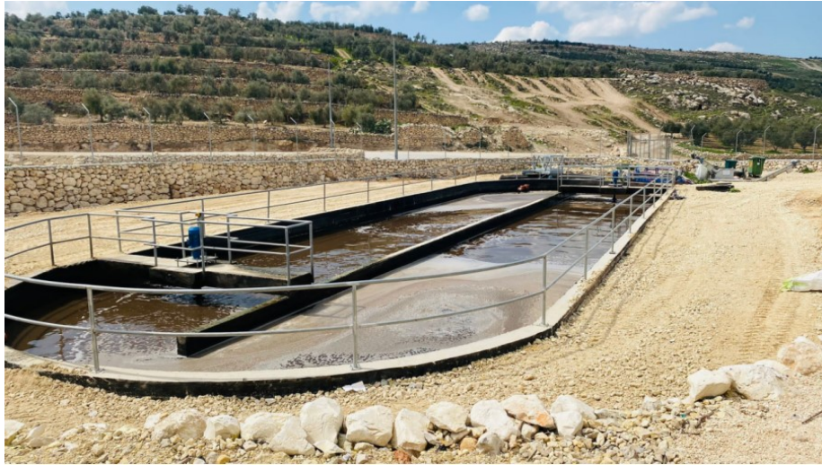
Figure 6: Picture of the WWTP of Kharas town (aeration tank for the biological treatment).
