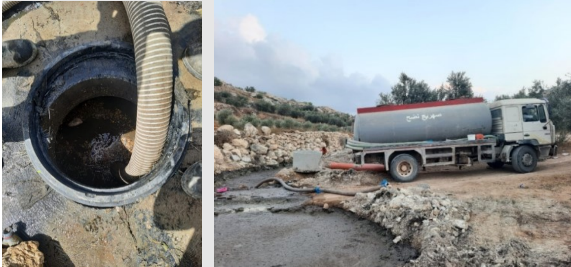
Figure 11: Septic tank being emptied and an example of dumping the faecal sludge (Wadii) (Municipality of Nuba).
