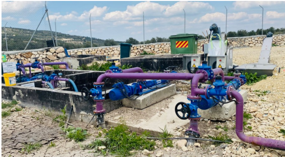
Figure 7: Picture of the WWTP of Kharas town (screening and sludge line).
