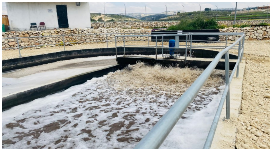
Figure 8: Picture of the WWTP of Kharas town (mechanical aerator).
