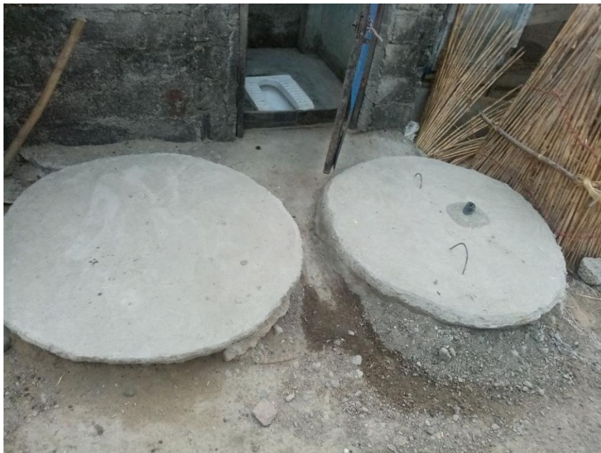
Figure 4: Inappropriate design of a twin pit.
