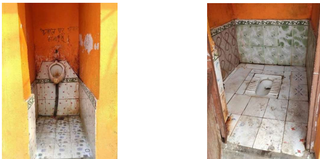
Figure 16: Status of urinals and pans of toilet at Ganga Sagar .
