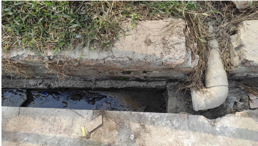
Figure 28: Outlet of a containment connected to an open drain found during field observation at Janakpurdham Sub-Metropolitan City.
