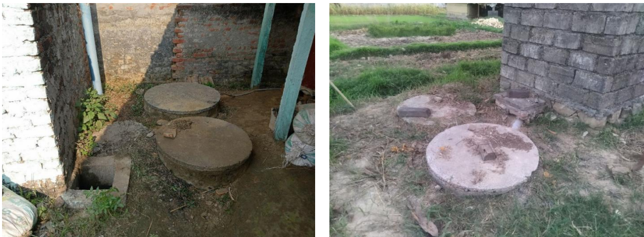
Figure 7: Inappropriate design of twin pits, the distance between two pits is less than 1.2m.
