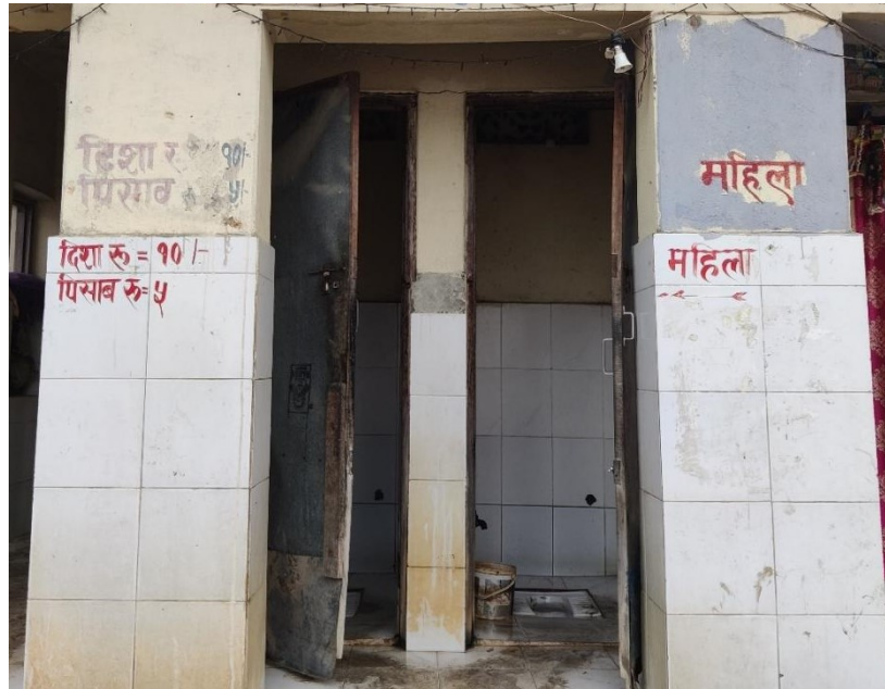
Figure 11: Status of the public toilet at Ramananda Chowk .
