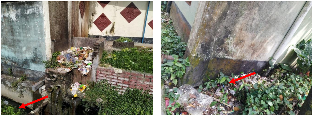
Figure 6: Containment system and their connections Left: Toilet Pit open to drain, Right: Toilet pipe connected to open environment (Source: Feasibility study 2020-21/DPHE).
