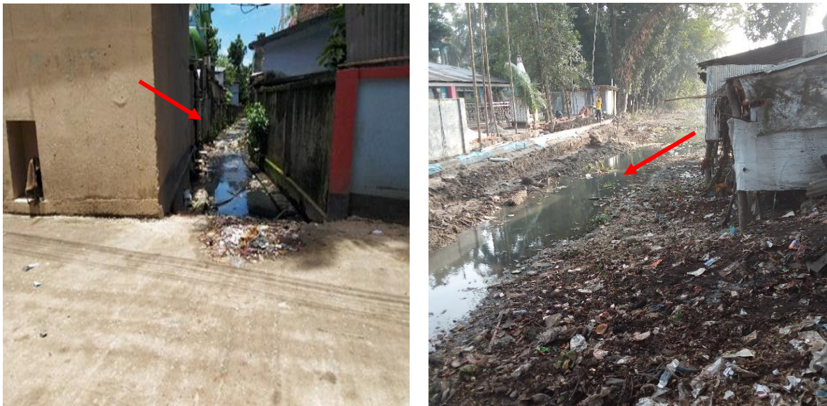
Figure 6: Containment technologies and their connections in Habiganj. Left: Toilet Pit open to a nearby water body, Right: Toilet pipe connected to open environment. (Source: Feasibility study 2020-21/DPHE).
