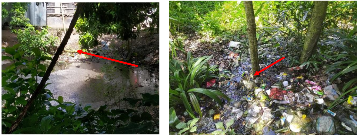
Figure 6: Containment technologies and their connections in Narail. Left: Toilet Pit open to a nearby water body, Right: Toilet pipe connected to open environment. (Source: Feasibility study 2020-21/DPHE ).
