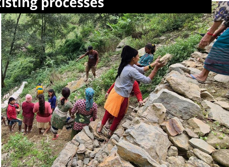
Community members create a wall from local materials to protect their water source – SNV Nepal/ Heman Paneru
