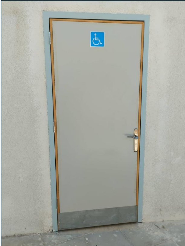
Figure 6: Door of constructed toilet for PWD (source internal from S4M in Jordan in 2022)
