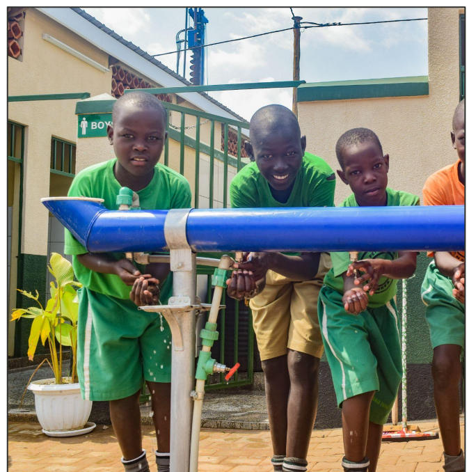
Top: a WASHaLOT 3.0 installed outside a school toilet block in Kampala; Bottom: Students washing their hands at a WASHaLOT 3.0 handwashing station.
