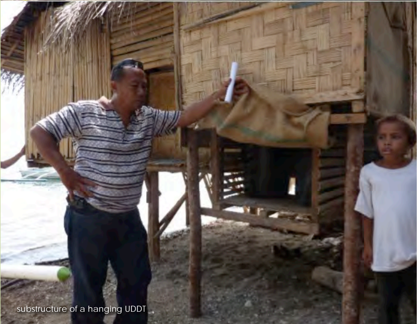
hanging UDDT attached to a coastal house in Initao, Misamis Oriental
