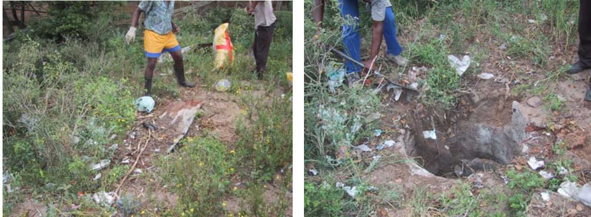
The pit as it was discovered in 2003. The tin sheet has been removed and the top ring collapsed. There are plans to refit another top ring, cast a new slab and put the pit back into use.
