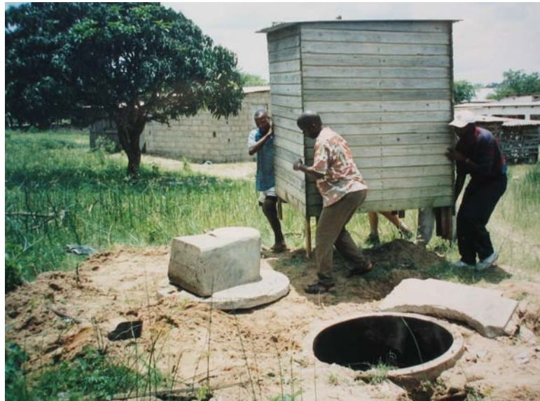
The 200 litre drum has been covered with the slab and pedestal and the superstructure is now being fitted (2000).
