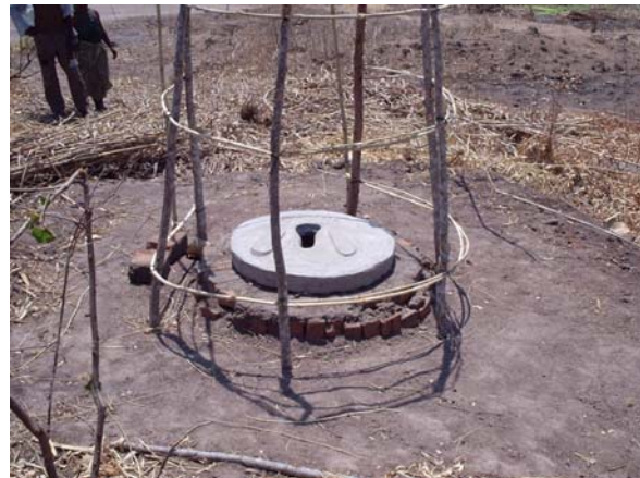
Slab mounted over pit with ring beam (Phalombe) Early stage for Arborloo
