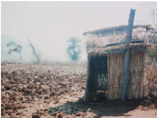
VIP latrines can also be low cost too! It works perfectly
