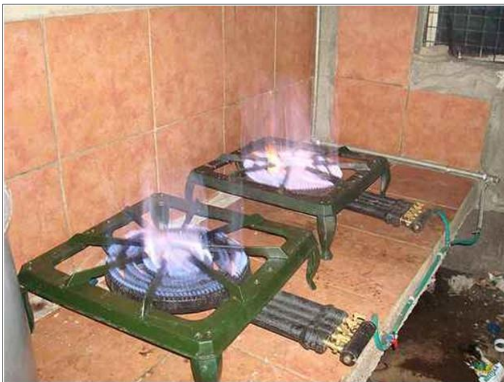
Pic. 23: Biogas being used in a cooker in a girls high school (source: GTZ).
