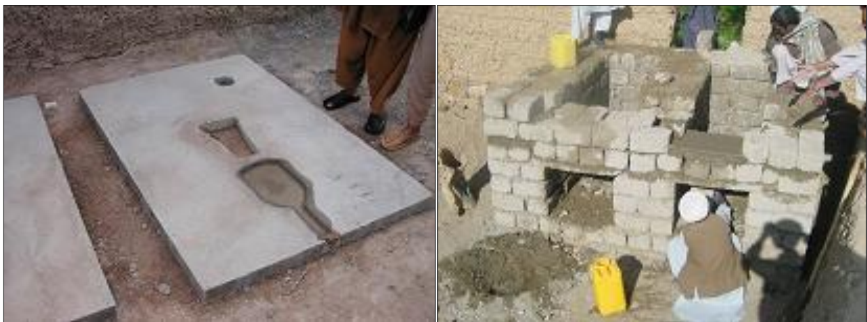
Pic. 19 - 20: Left. Moulded concrete slab of a urine-diverting toilet made by the women’s committee. Right. The substructure of a double vault UDDT in the Clean Village Project (source: VWO, 2009).
