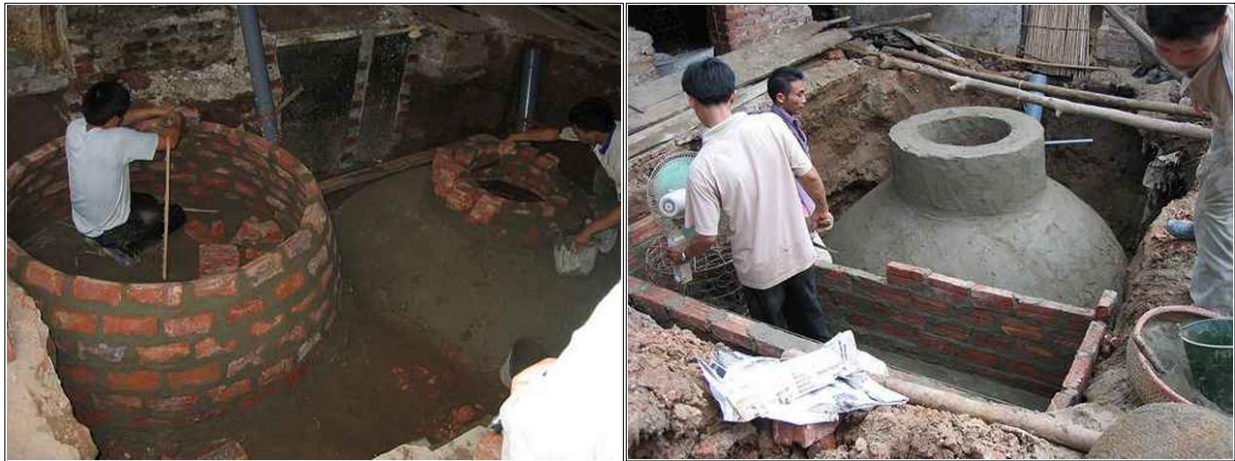
Pic. 21 - 22: Construction of a fixed-dome biogas digester near Hanoi, Vietnam (source: GTZ).
