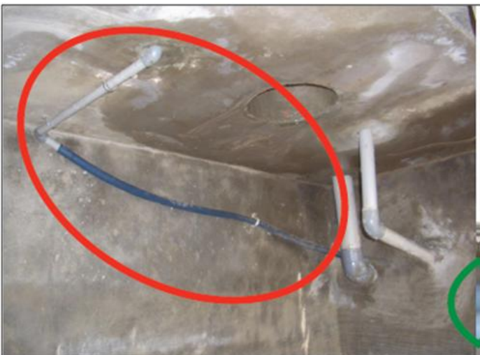
Pic. C5: Urine collection pipe too narrow and too many bends
