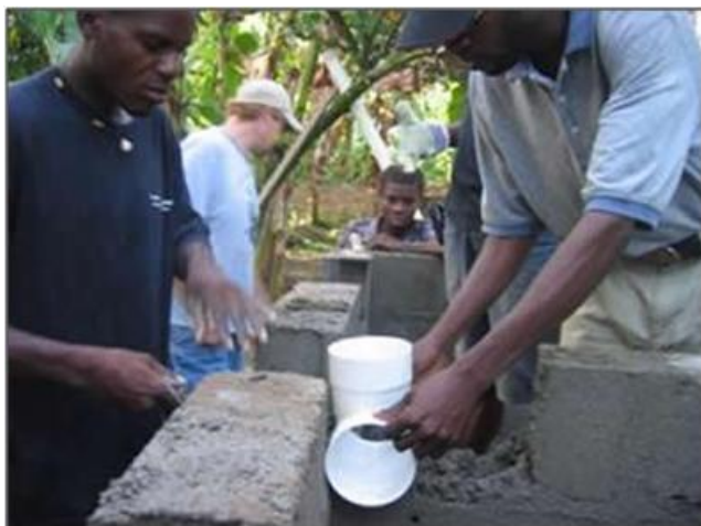
Pic. C1; Placement of the bifurcating ventilation pipe in a double vault toilet.
