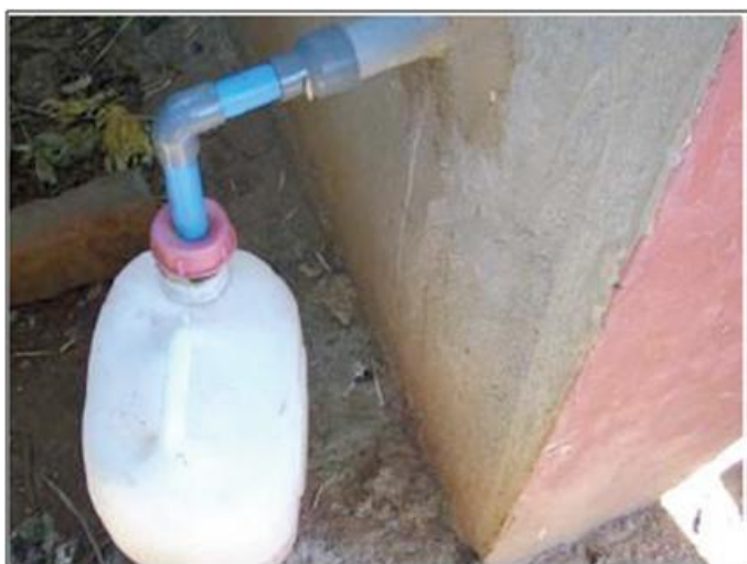
Pic. C2: Connection of urine collection pipe to sealed urine container
