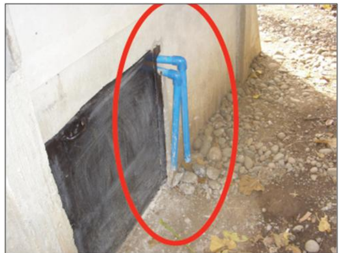
Pic. C6: Improper discharge of washing water
