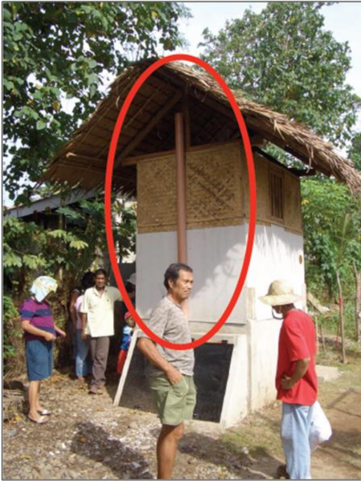
Pic. C4: Ventilation pipe too short. It should extend 20 - 30 cm above the roof.
