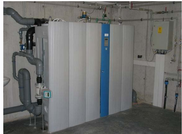
Figure 2: PONTOS Aquacycle 1500, SBR greywater treatment
