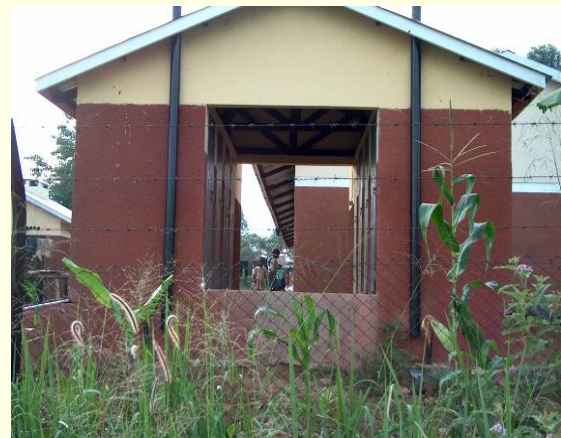
Figure 1: Urine diverting dry toilets in Maracha Hospital.
