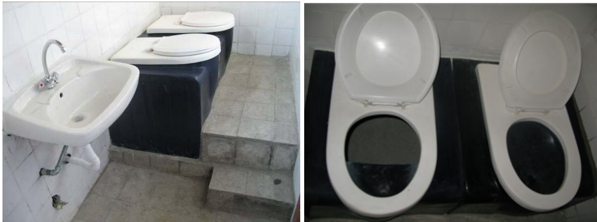
Figure 2: Double vault system in the bathroom
