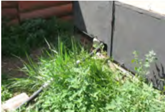
Figure 8: Conducting urine into the former pit-latrine.
