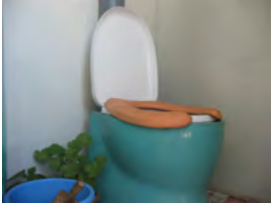
Figure 7: Inside view of ECOSAN-toilet with ashes-bowl.
