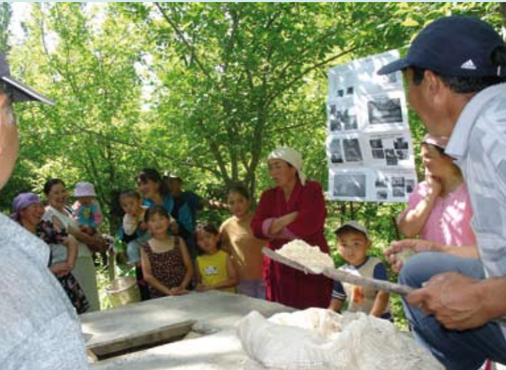
Interested neighbors visit the construction site of a UDDT in Kerben, South Kyrgyzstan. The opportunity is used for information and training by PA ULGU.
