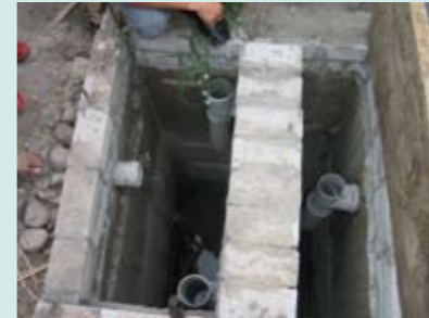
Sedimentation tanks of Ivanovka constructed wetland.
