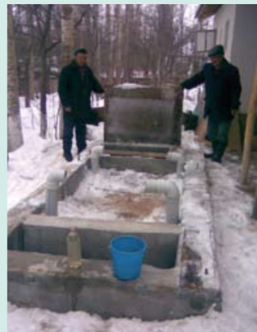
Constructed wetland in Jetygen. The filter never froze even at outside temperatures of -20°C.
