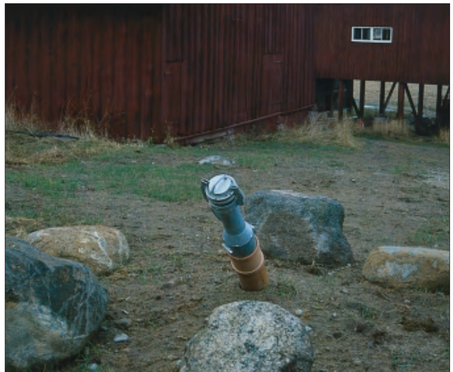
Connection pipe used by tank trucks to fill the storage tanks at Lake Bornsjön.
