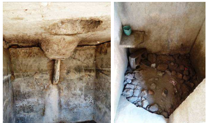
Fig. 9: Situation 8 years after construction: Left: walls of faeces vault with deep cracks. Right: bathing cubicle's concrete floor is broken (source: A. Leitner, 2011).
