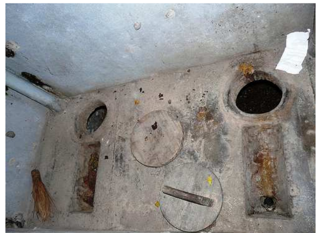
Fig. 6: Very dirty and not well maintained UDDT (inside), 8 years after construction. It seems that both faeces vaults are used at the same time. Note the two round wooden lids to cover the faeces holes (source: A. Leitner, 2011).
