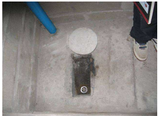
Fig. 5: Inside a new UDDT; the faeces hole is covered with a lid; the urine separation part is fitted with a sieve. You can see the ventilation pipe at the back left (source: M. Fogde, 2003).
