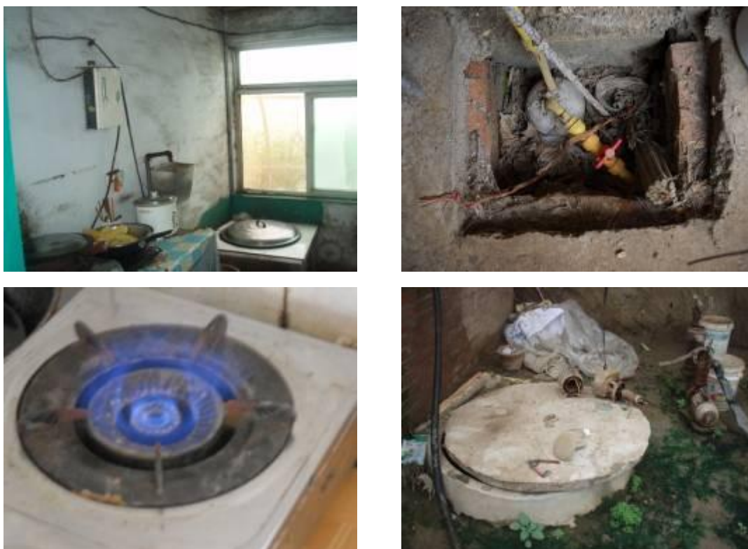
Figure 17: Biogas system components
