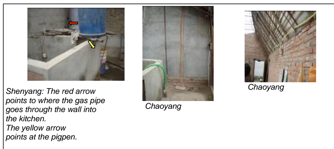
Figure 18: Outside gas pipelines
