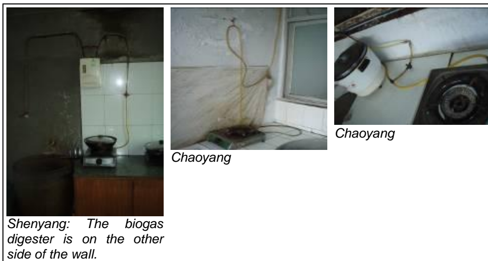
Figure 19: Inside gas pipelines
