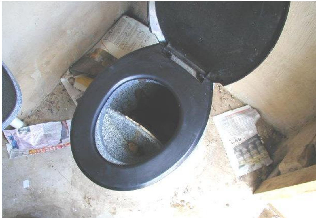
Figure 2: Poorly maintained UD Toilet (source: Holden, 2004)
