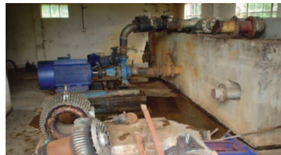
Dysfunctional pump room
