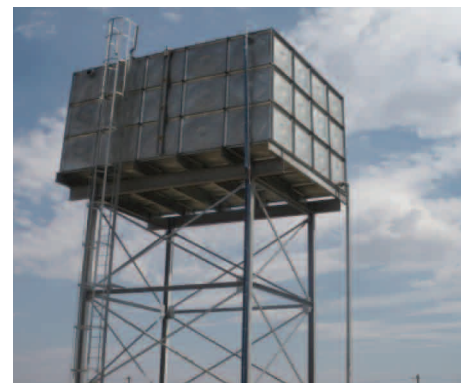
Treated grey water storage tank
