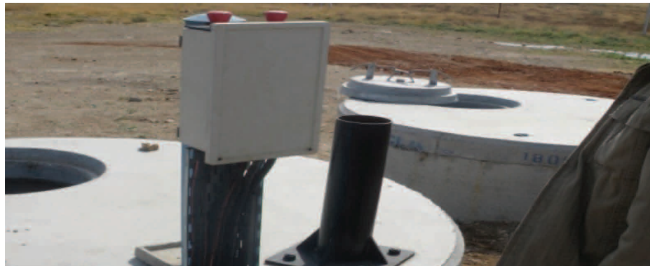
Two manholes that receive wastewater from households
