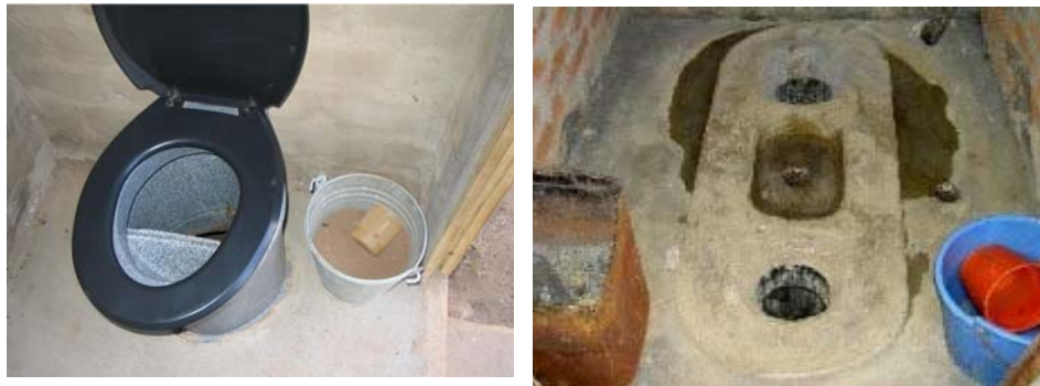
Figure 3-2 Urine Diverting Toilets, a Pedestal Type (left) and a Squat Type (right) with a Third Hole (at the back) for “Washers”.
