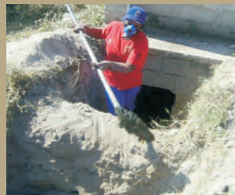
Fig. 10: Formalised pit emptying in eThekweni © Jay Bhagwan
