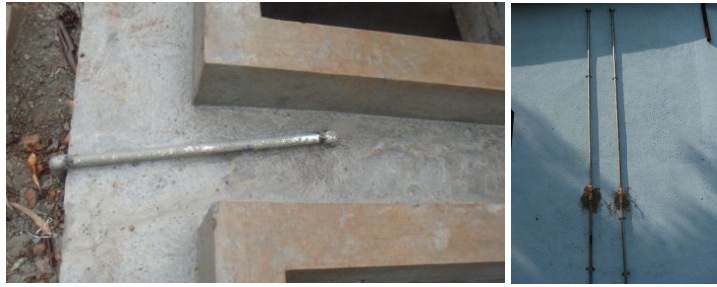
Pipeline collecting biogas from ABR
