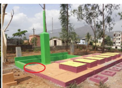
Outlet of Anaerobic Filter (AF)
