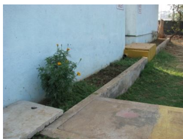
Inlet (pipeline from toilet block)
