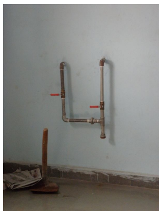
Visible water trap
