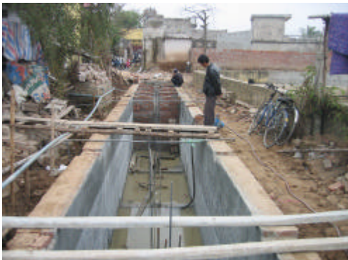
Figure 3. BASTAF under construction for a group of 80 households in Lai Xa commune, 20 km from Hanoi centre (photo by Nguyen V. A., 2006)
